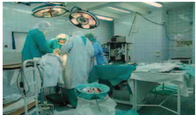
Air Conditioning of surgical operating room
